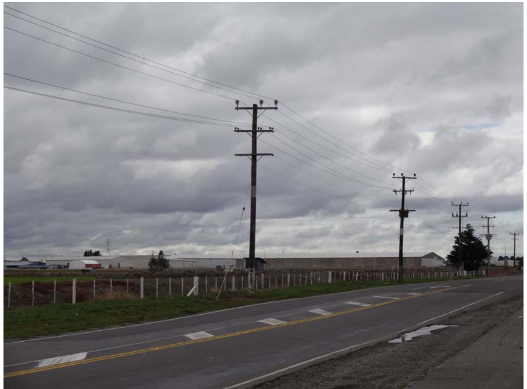
Photo 3 – 33kV line in a developing residential/industrial zone
